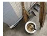
Equipment for container inspection.jpg
